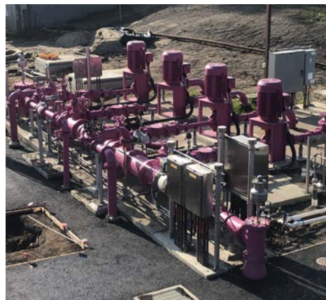
New Recycled Water Distribution Pump Station
