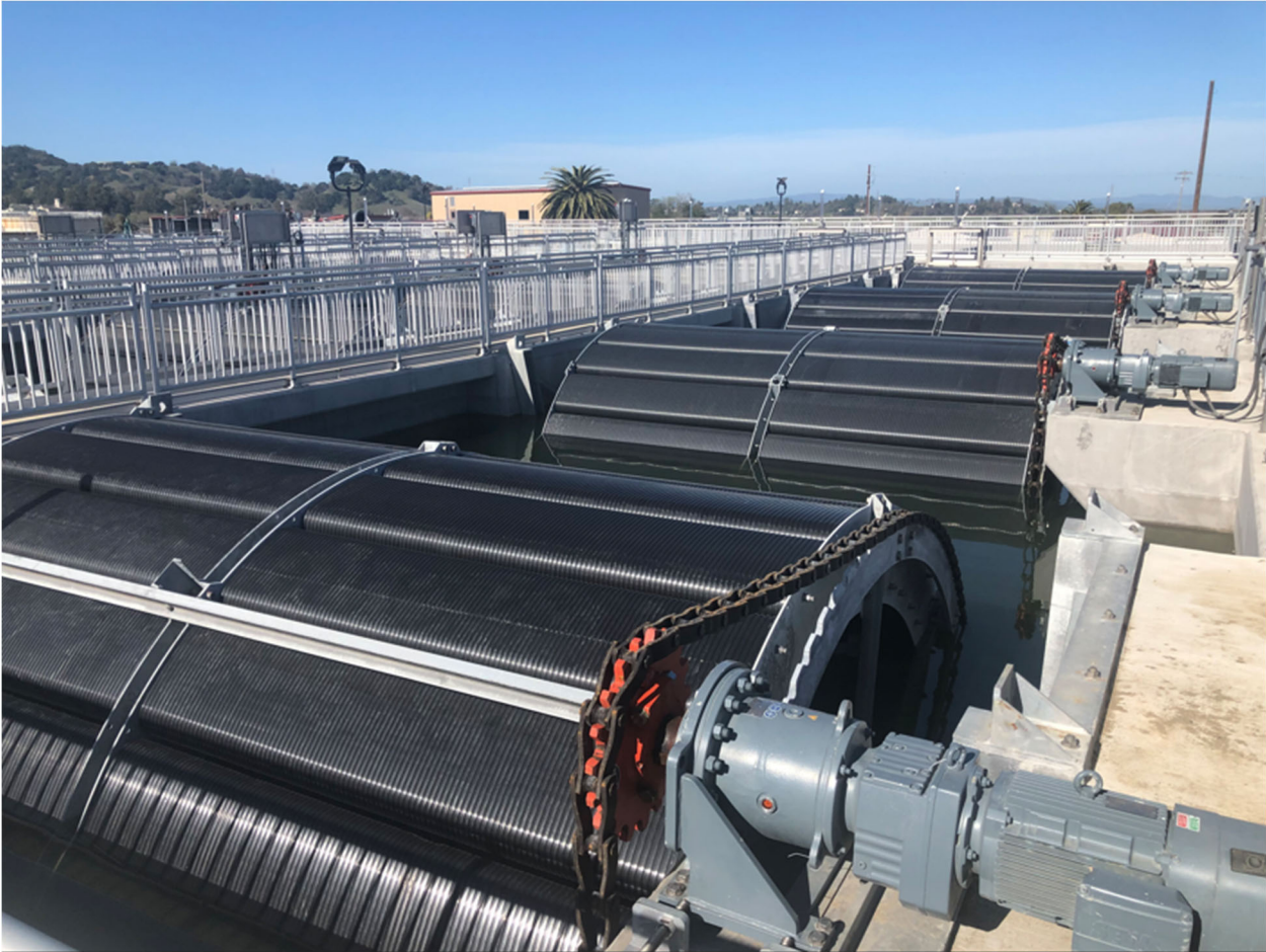
Biowheel aeration system
