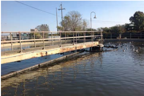
This is the LGVSD secondary clarifier, which has been in service continuously since 1964 at the wastewater treatment plant. The clarifier will require significant modification to work with the other planned improvements.
