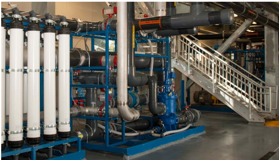
Las Gallinas' reverse osmosis filtering equipment is just one step in the advanced treatment of wastewater.
