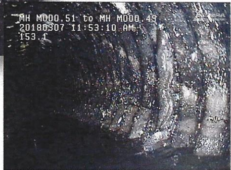
153' Faulty joint seal
