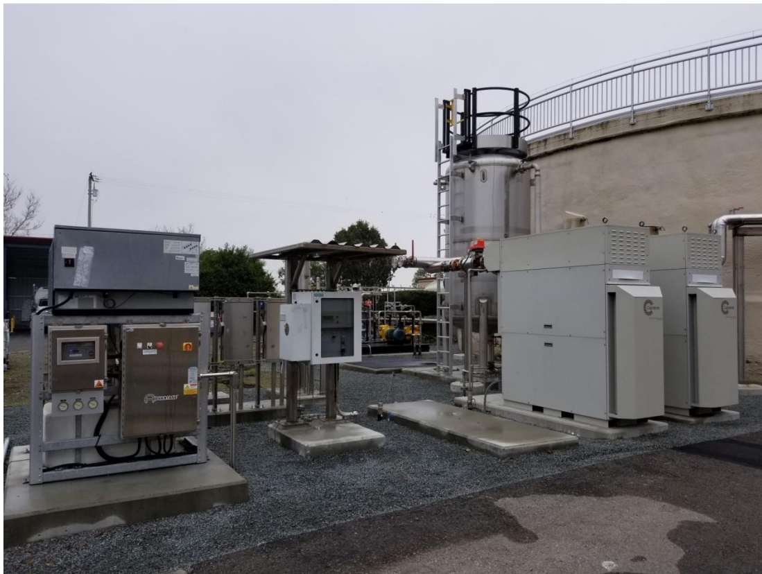
Biogas Recovery System Microturbines
