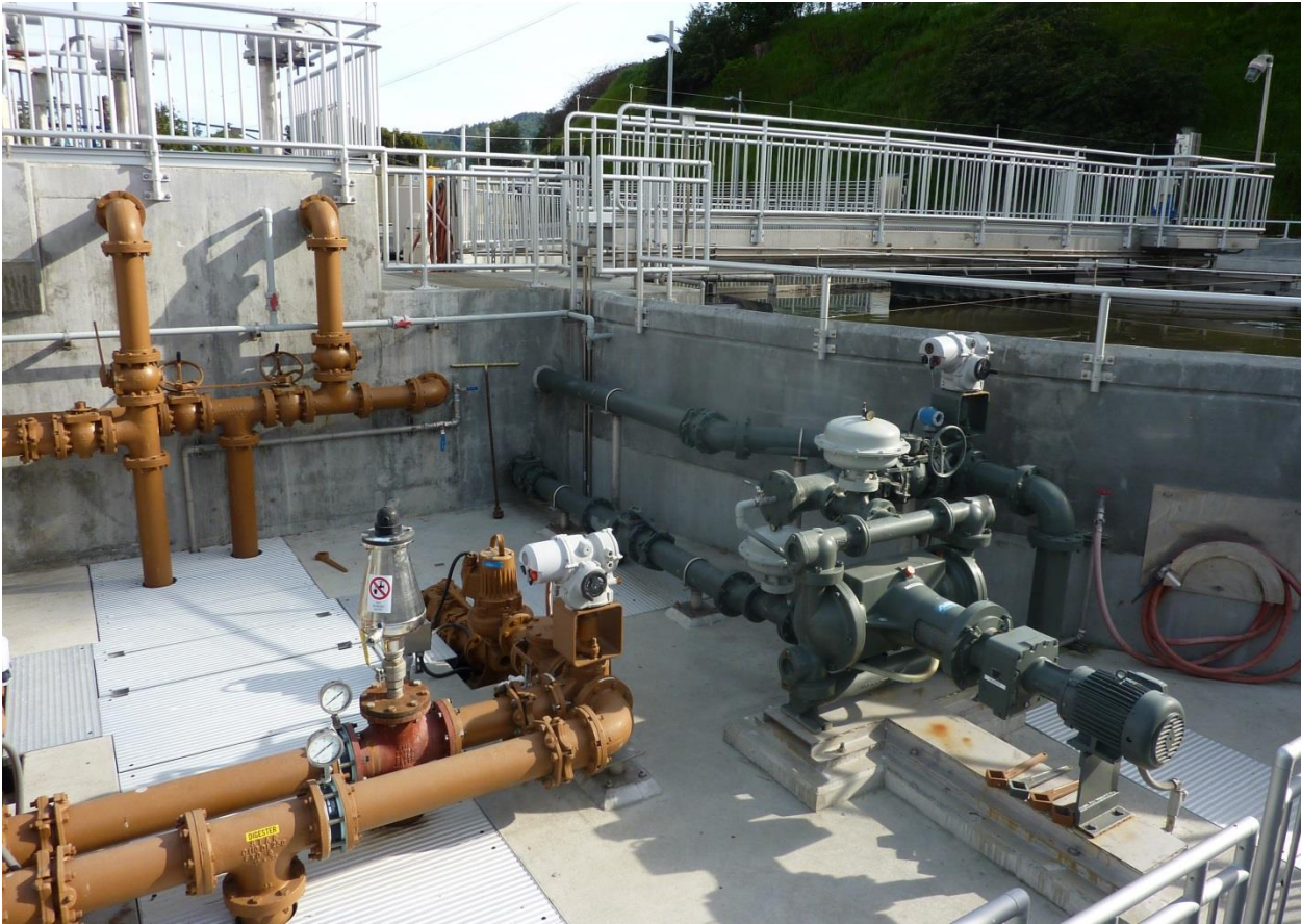
Primary clarifier sludge pump facilities
